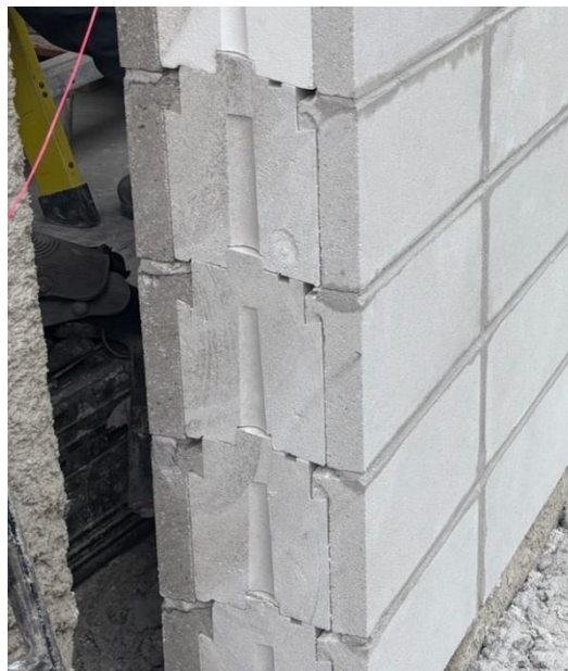
Example of overlap and continuity of insulation after cutting the rough opening
